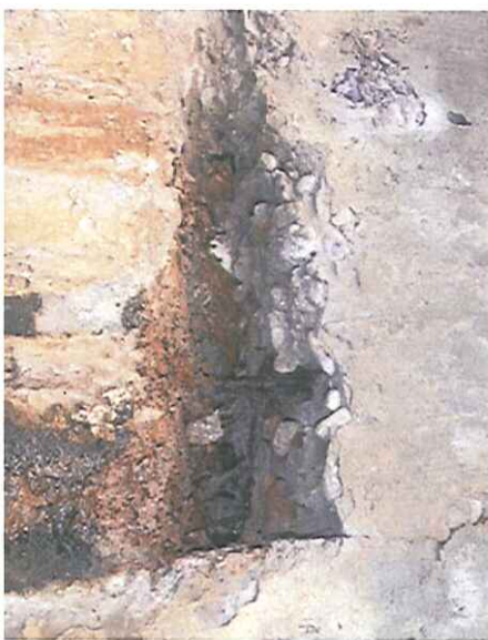
Figure 1-26: Spall with exposed rebar at left end abutment upstream wingwall.
