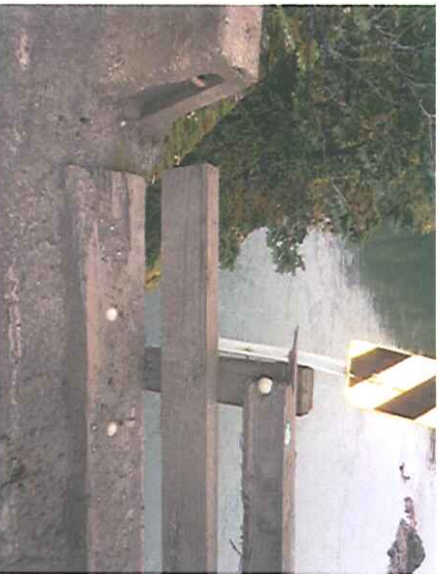
Figure 1-15: Damaged downstream handrail near left end.
