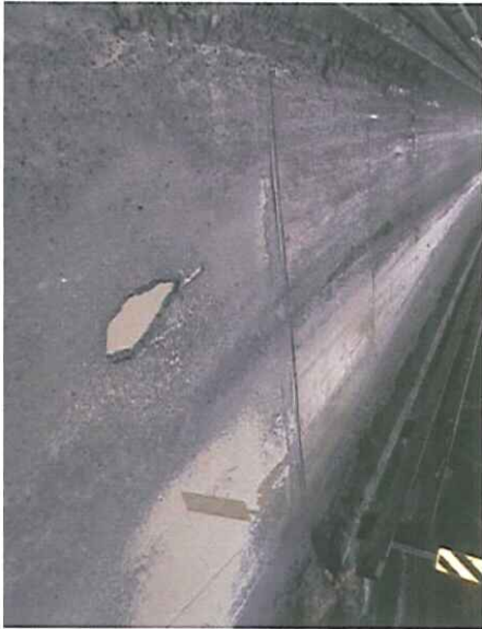
Figure 1-7: Left end approach joint - note pothole.
