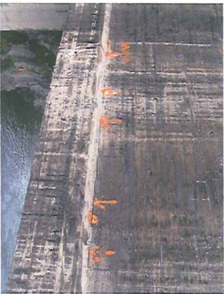
Figure 1-18: Girder 1 u/s face - check along bottom flange near left abutment. See notes.
