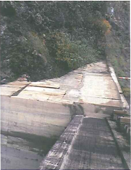
Figure 1-24: Left end abutment upstream wingwall - note concrete deterioration & water ingress.
