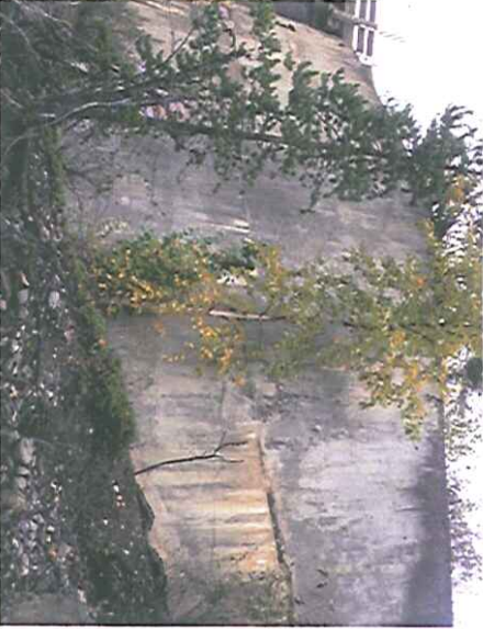
Figure 1-29: Right end abutment upstream wingwall - note concrete deterioration.
