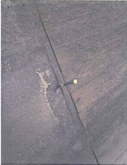
Figure 1-8: Left end approach joint - note failed armoring.
