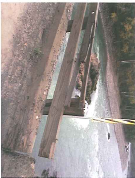
Figure 1-14: Damaged upstream handrail and post near left end.
