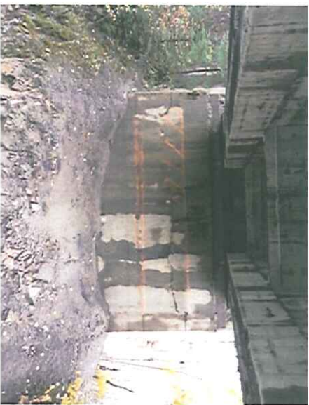
Figure 1-28: Front face of right end abutment. note delamination.
